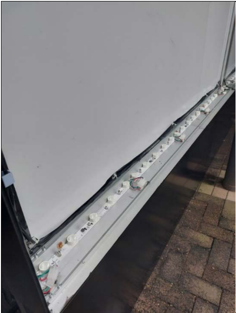
LB2 (Internal light fittings)
